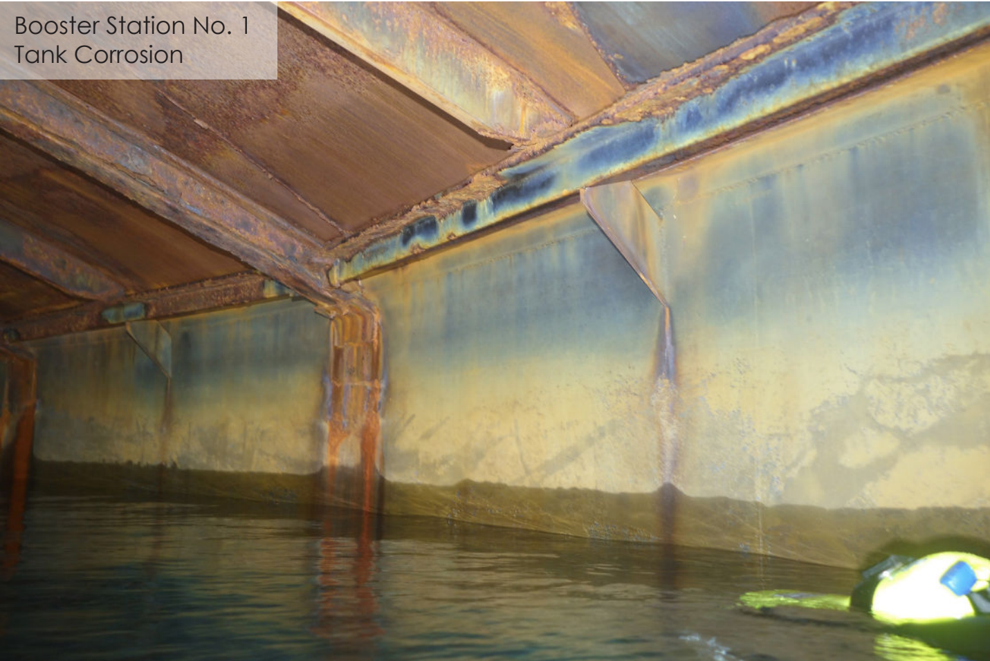
Booster Station No. 1 Wall Corrosion
